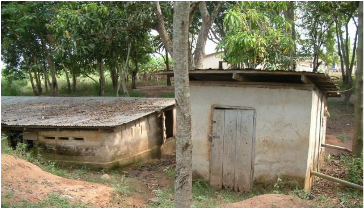
Figure E2: Existing spring box (left) and pump house (right). Notice the existing piping from the right side of the pump house.
